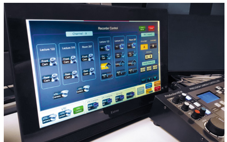
The support team uses an Extron TLP Pro 1520TG TouchLink Pro 15" capacitive touchpanel to manage all AV operations from the control room.
